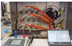
Insulation resistance test
